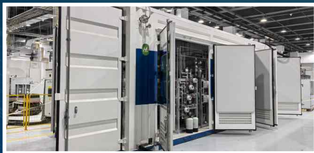
◀ Skid-Mounted PEM Hydrogen Production Project ▶
