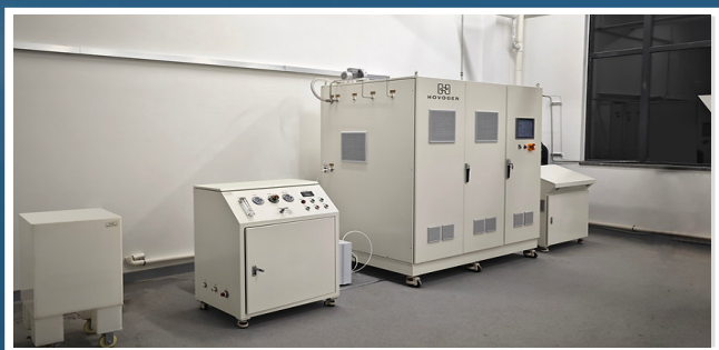
◀ 35MPa High-Pressure Hydrogen Production Project ▶
