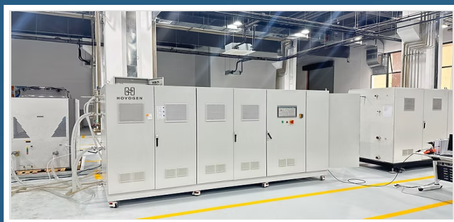
◀ Semiconductor Hydrogen Supply Project ▶
